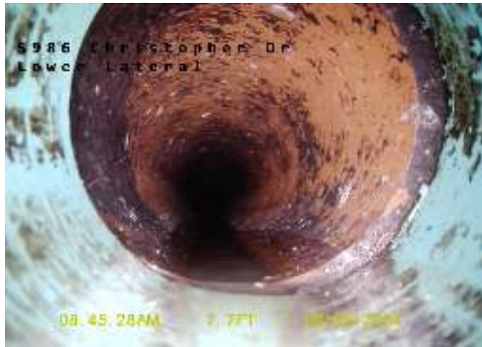
Figure 1: Photo of offset in lower lateral of 5986 Christopher Dr. as recorded on August 5, 2024
