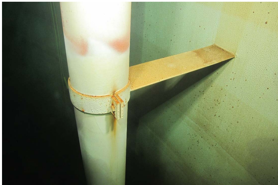
I-49 Same as Photo I-48, except further up the overflow. Note corrosion on the stand-off bracket.
