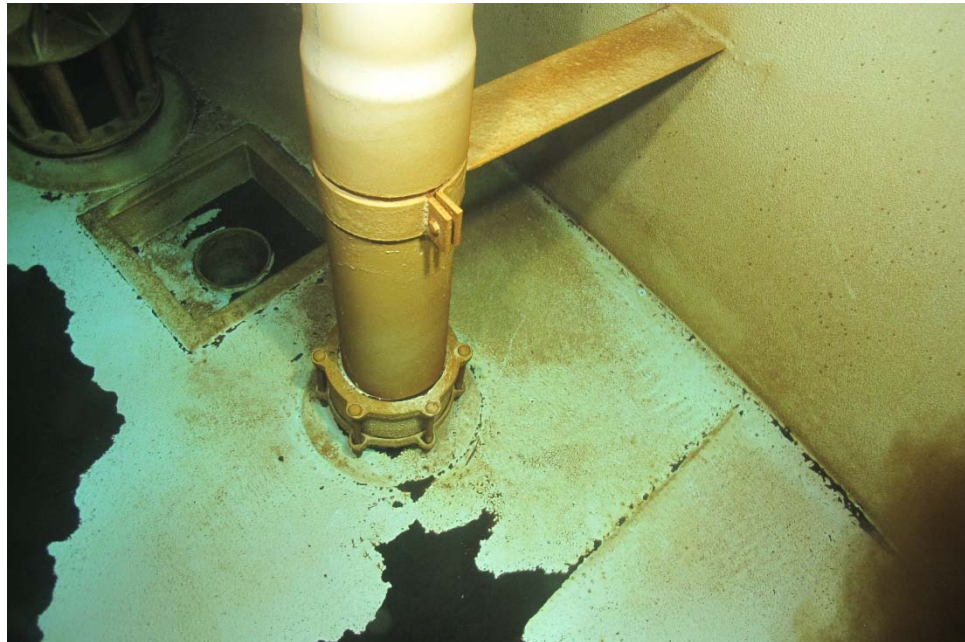
I-48 View of the overflow, illustrating blistering of the coating system on the stand-off bracket and compression flange.
