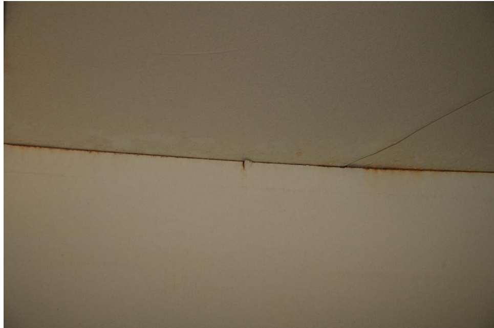
I-18 Same as Photo I-17, except a close-up view of the transition. Note small spot of cracked coating.
