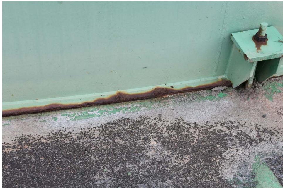
E-27 View of the bottom plate extension (BPE), illustrating moderate to severe corrosion along the edge of the BPE. Note areas where corrosion is encroaching on the shell to BPE weld.
