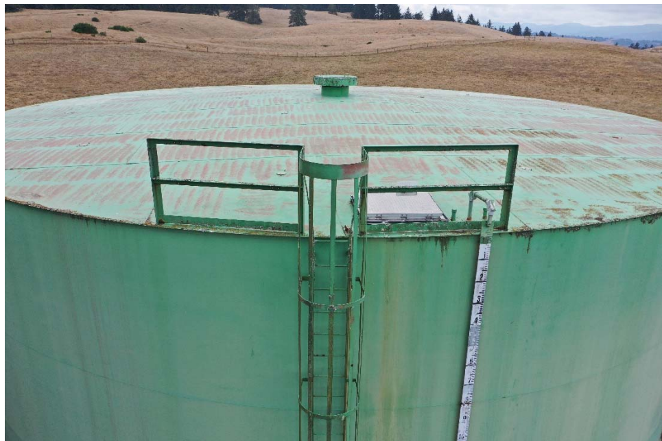
E-13 View of the top of the ladder, illustrating exposed prime coat on the ladder cage.
