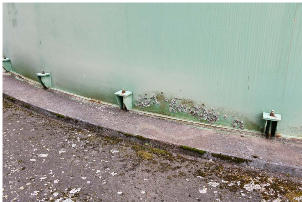
E-25 View of seismic anchor bolts, illustrating moderate corrosion on the nuts and bolts and moss along the lower portion of the shell.
