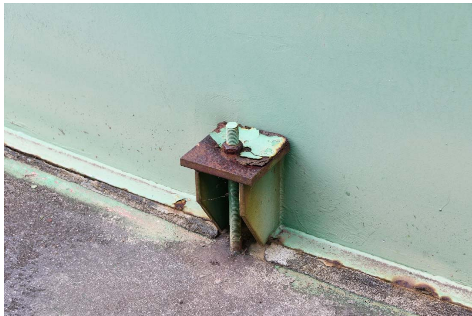
E-26 Same as Photo E-25, except a close-up view of an anchor bolt. Note moderate to severe corrosion with delaminating paint on the anchor chair.
