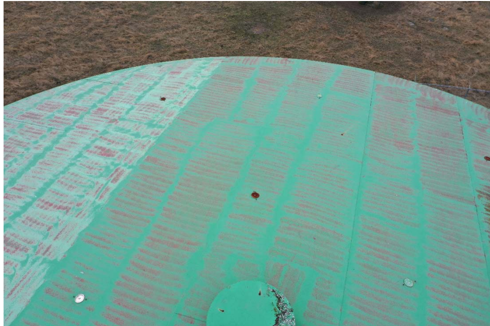
E-6 Same as Photo E-5, except in a different location. Note general corrosion on the handhole covers.
