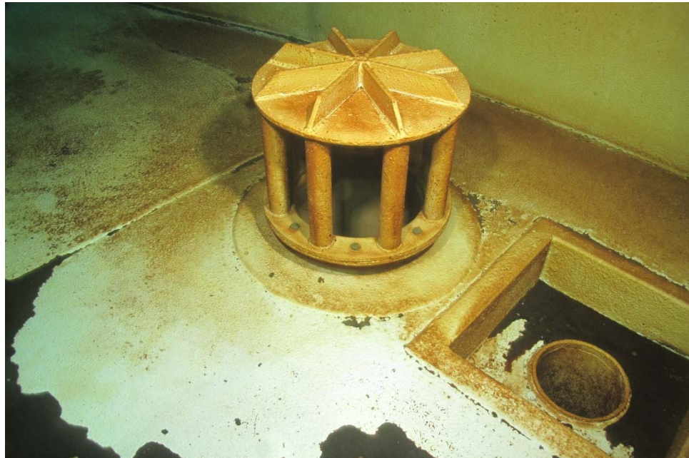
I-51 View of the inlet/outlet diffuser, illustrating blistering of the coating system.
