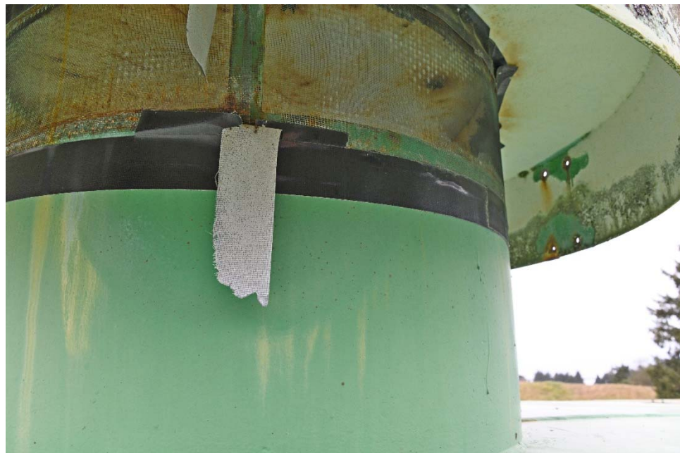
E-4 View of the underside of the center vent cover, illustrating minor to moderate corrosion on the vent cover, neck, and screening. Note failing tape securing the vent screen.
