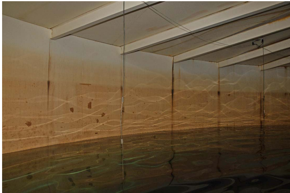
I-19 View of the shell, illustrating staining in the water fluctuation zone and otherwise good condition of the coating system.
