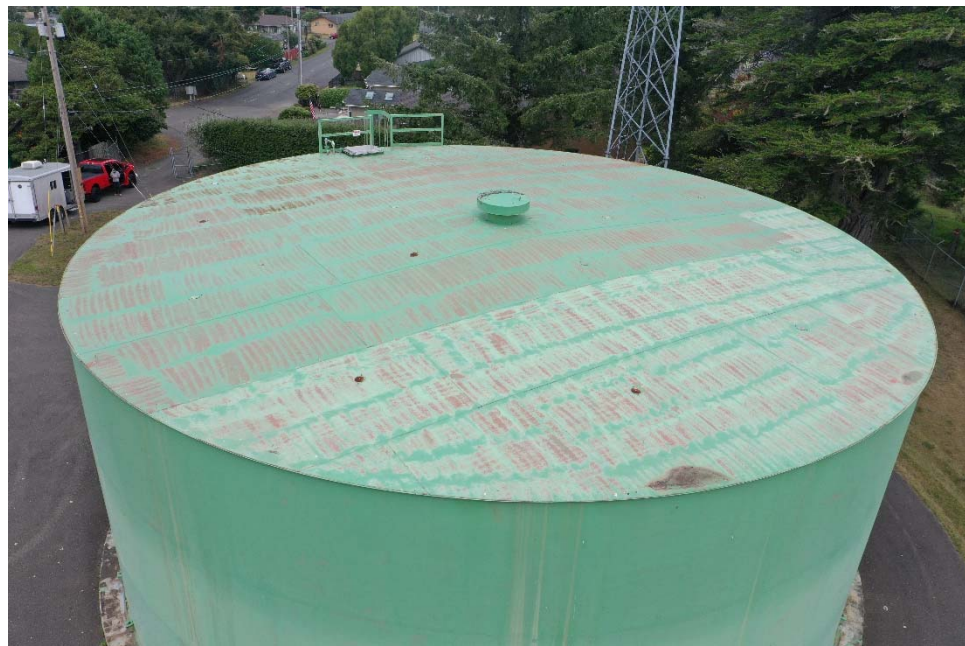
E-2 Same as Photo E-1, except a closer view of the roof. Note pattern of exposed prime coat on the roof plates.
