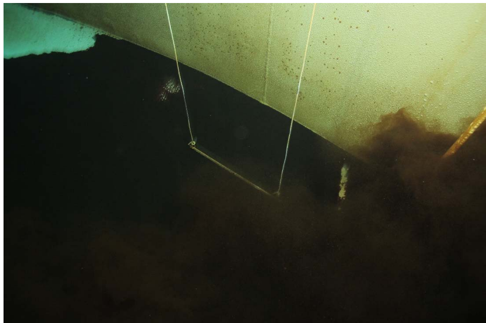
I-52 View of the LLI base, illustrating generally good condition of the base and guide wires.
