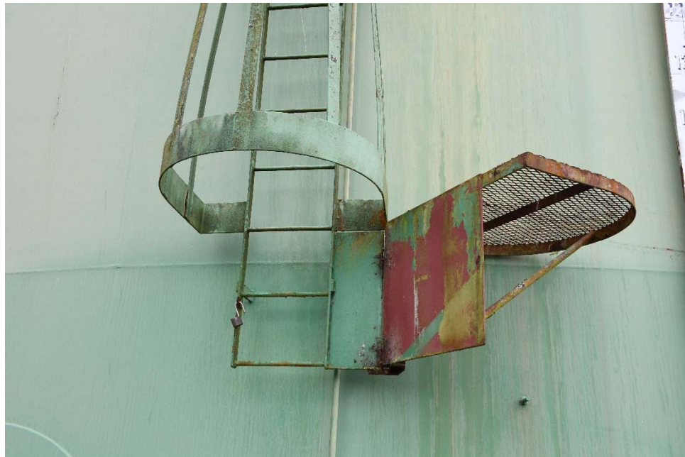
E-15 View of the ladder vandal guard, illustrating red primer on the vandal guard.
