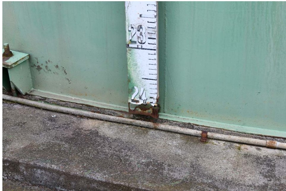
E-24 Same as Photo E-23, except at the bottom of the gauge board. Note severe corrosion at the bottom of the board.
