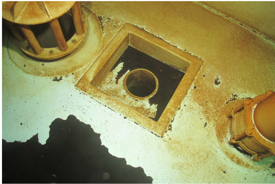
I-50 View of the drain sump and adjacent appurtenances, illustrating blistering of the coating system on all surfaces.
