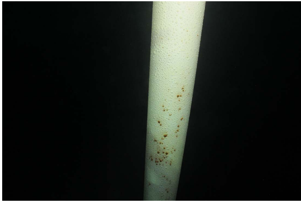
I-41 View of the column, illustrating blistering of the coating system with random spots of corrosion.
