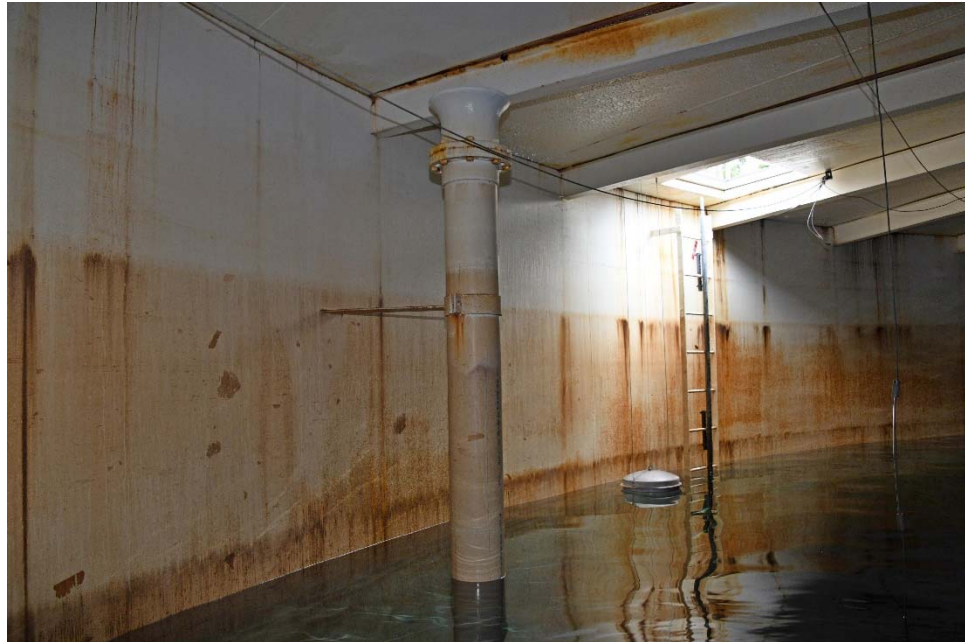
I-21 View of the overflow, illustrating corrosion at the upper flanges and stand-off bracket.
