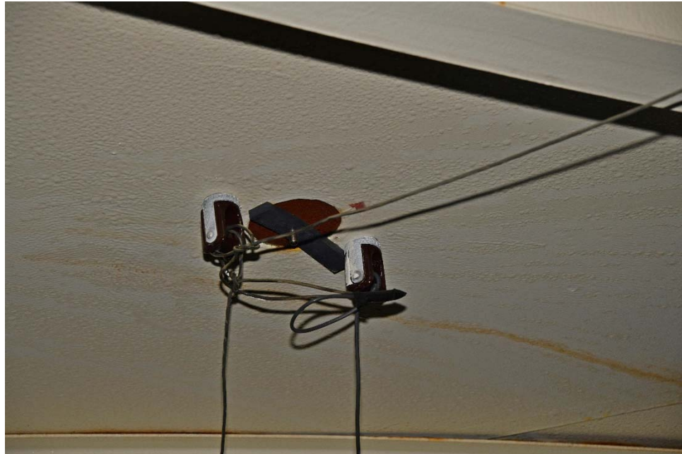
I-12 View of a cathodic protection handhole, illustrating minor corrosion along the circumference of the handhole and oxidation of the adjacent hardware.
