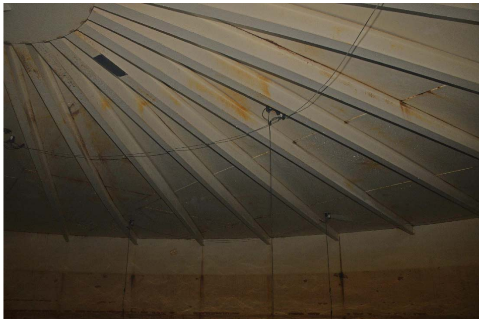
I-4 View of a portion of the roof, illustrating random general corrosion on the roof plates and rafters.
