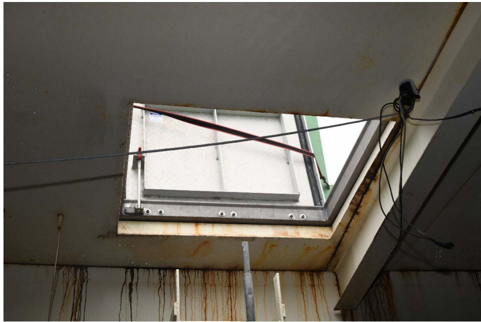
I-26 View of the roof hatch, illustrating minor corrosion along the perimeter of the hatch opening.
