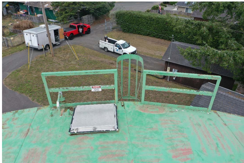
E-10 View of the roof hatch/work area, illustrating general corrosion and moss growing on the guardrail.
