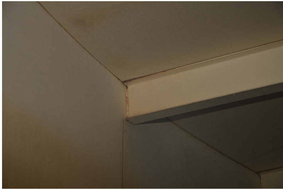
I-14 View of a rafter to shell connection, illustrating minor corrosion along the upper rafter flange and otherwise good condition of the coating system.
