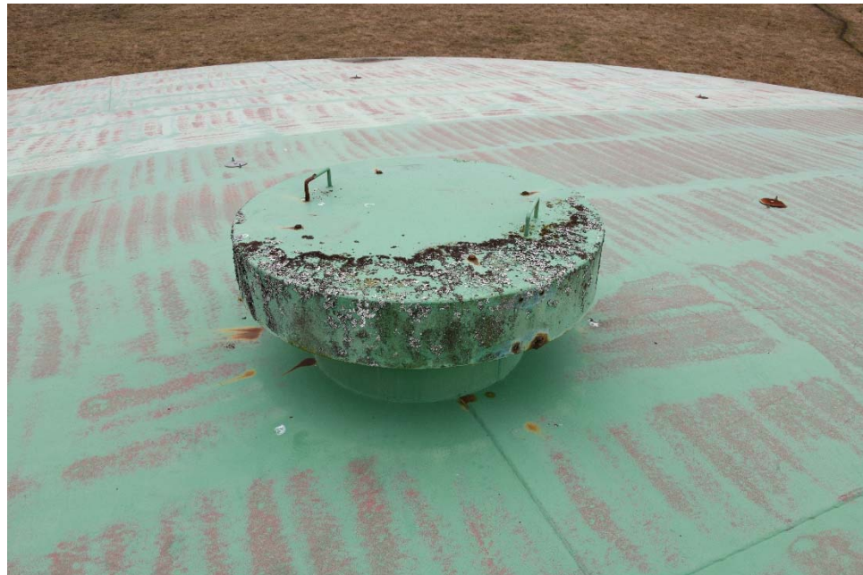
E-3 View of the center vent, illustrating moderate corrosion on the vent cover and nuts and bolts and moss growing on the cover.
