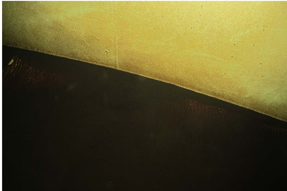
I-39 View of the shell to bottom transition, illustrating blistering of the coating system on the shell and dark sediment on the bottom plates.
