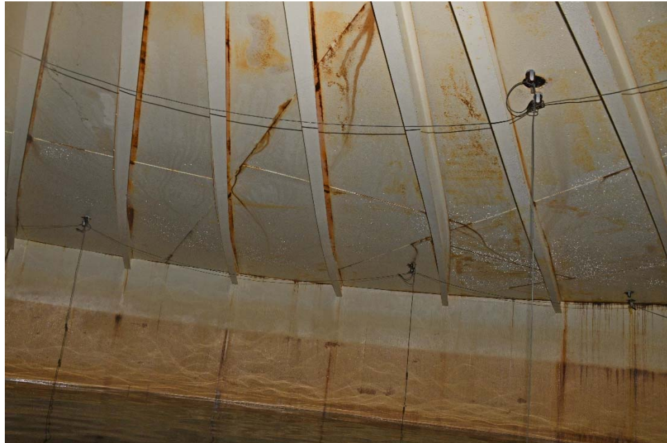
I-6 View of rafters, illustrating moderate to severe bowing and rolling of the rafters in this area.
