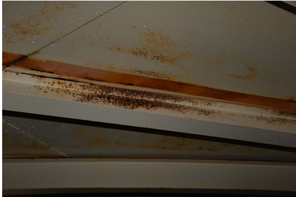
I-9 View of the roof above a rafter, illustrating general corrosion on the roof plates that previously rested on the rafter.
