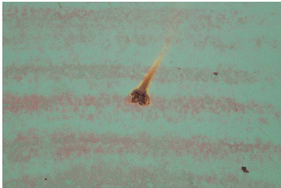
E-8 Close-up view of the roof, illustrating a spot of cracked paint with moderate corrosion.
