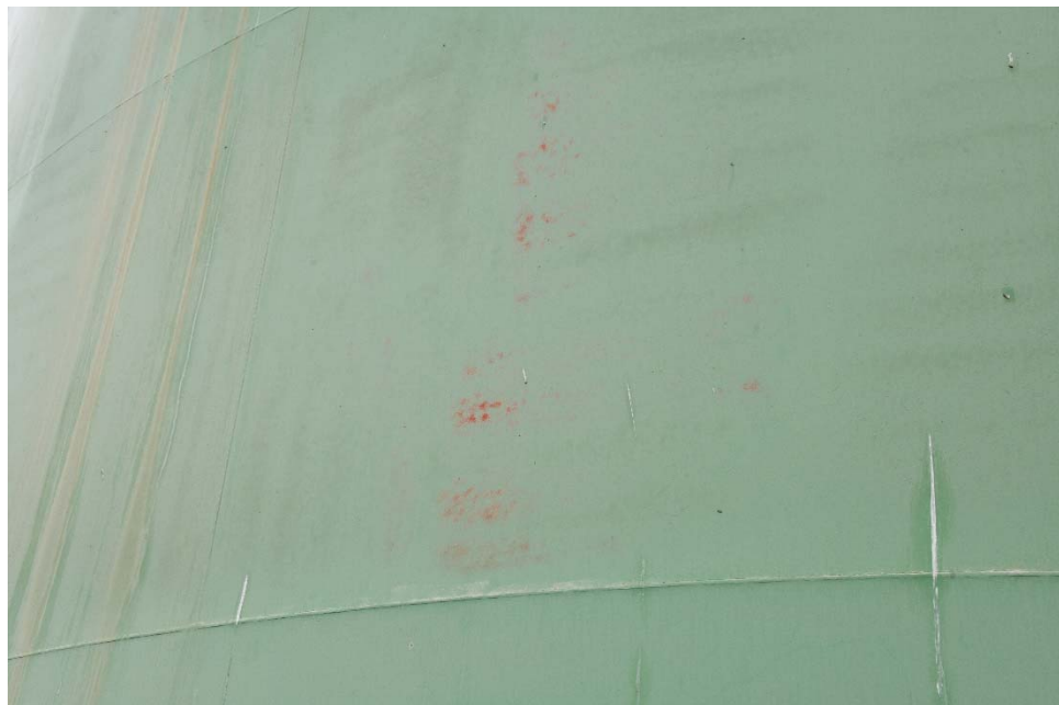
E-19 Same as Photos E-17 and E-18, except a closer view of the shell. Note areas of exposed prime coat.
