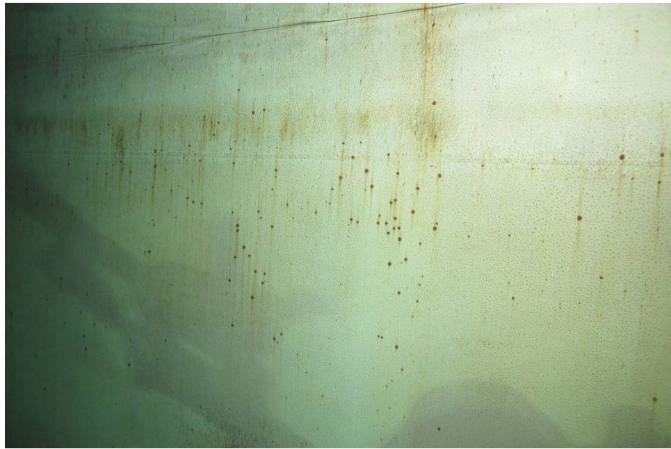
I-35 Same as Photos I-32 through I-34, except in a different location
