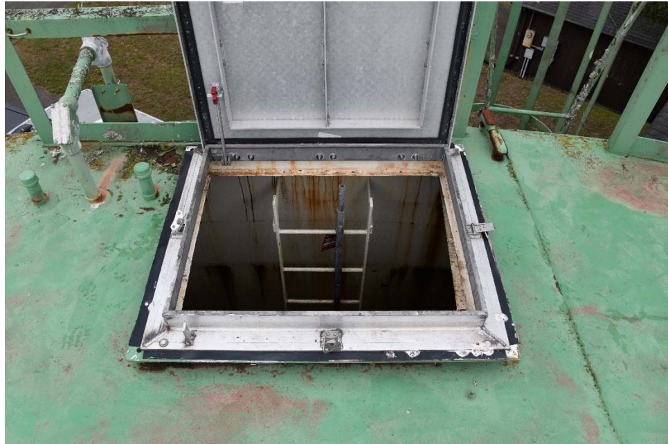
E-12 View of the roof hatch, illustrating minor corrosion along the perimeter of the interior of the hatch curb and good condition of the aluminum cover.
