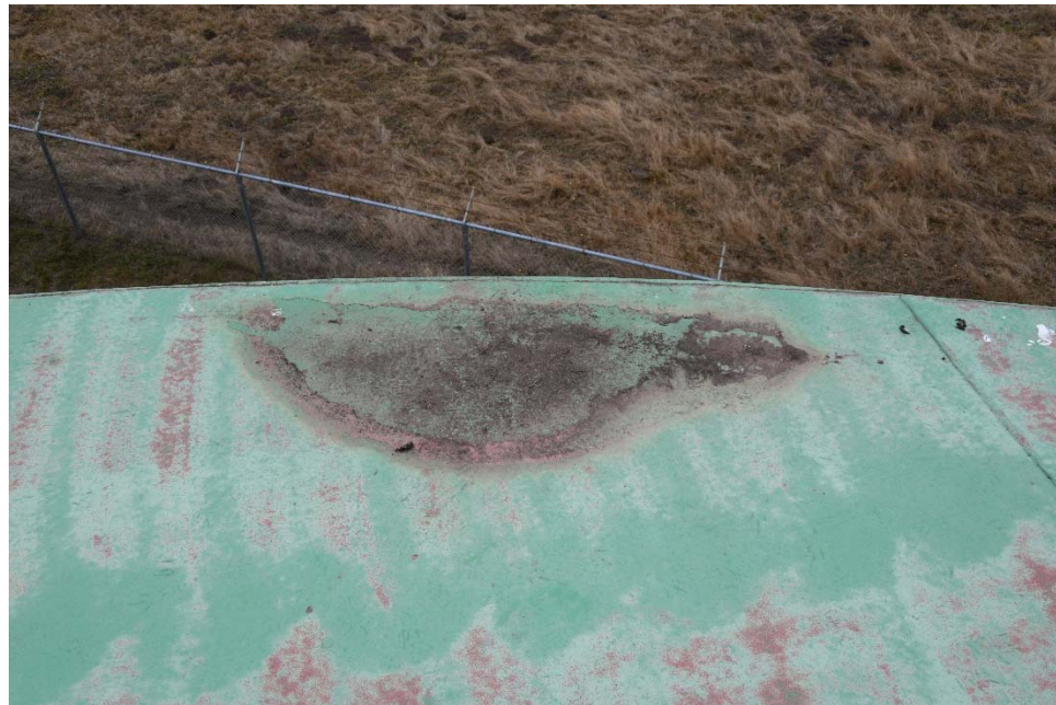
E-9 View of the edge of the roof, illustrating an area of dirt collecting at the edge of the roof with delaminating paint along the edges of the low area.
