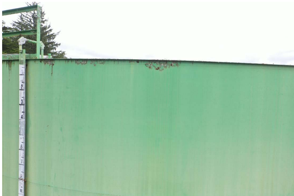
E-16 View of the top of the shell, illustrating moss growing under the top angle and otherwise generally good condition of the paint system.
