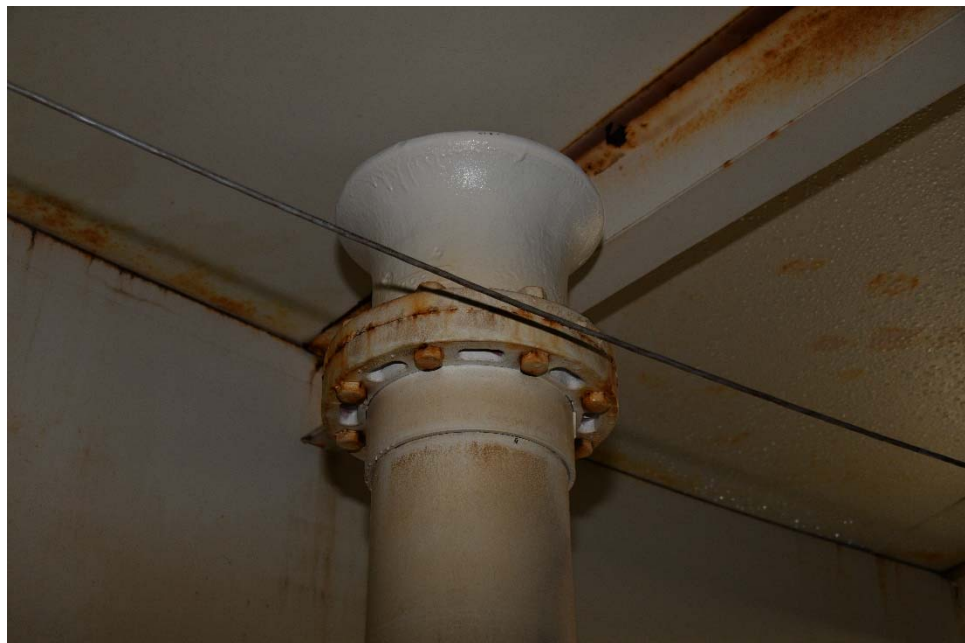
I-22 Same as Photo I-21, except a close-up view of the upper flanges.
