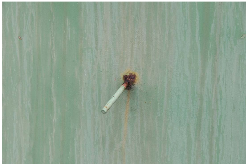
E-22 View of an abandoned bracket on the shell, illustrating moderate corrosion where the threaded rod meets the shell.
