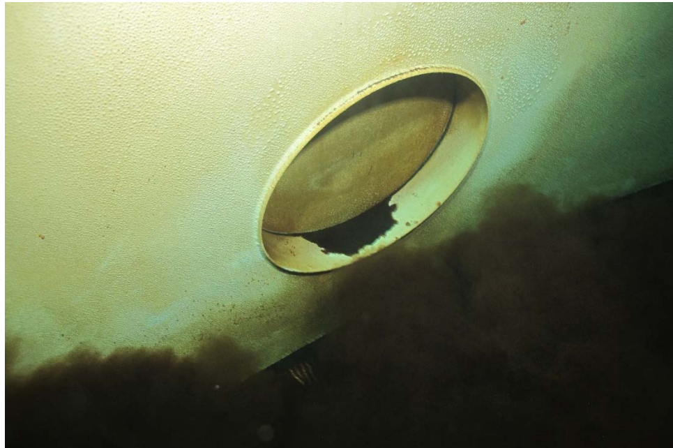
I-36 View of a manhole, illustrating blistering on the manhole cover, stiffener ring, and adjacent shell.
