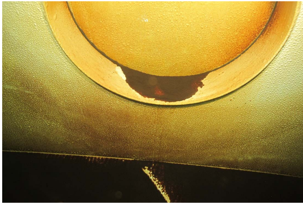
I-38 Same as Photo I-37, except a close-up view of the stiffener ring.
