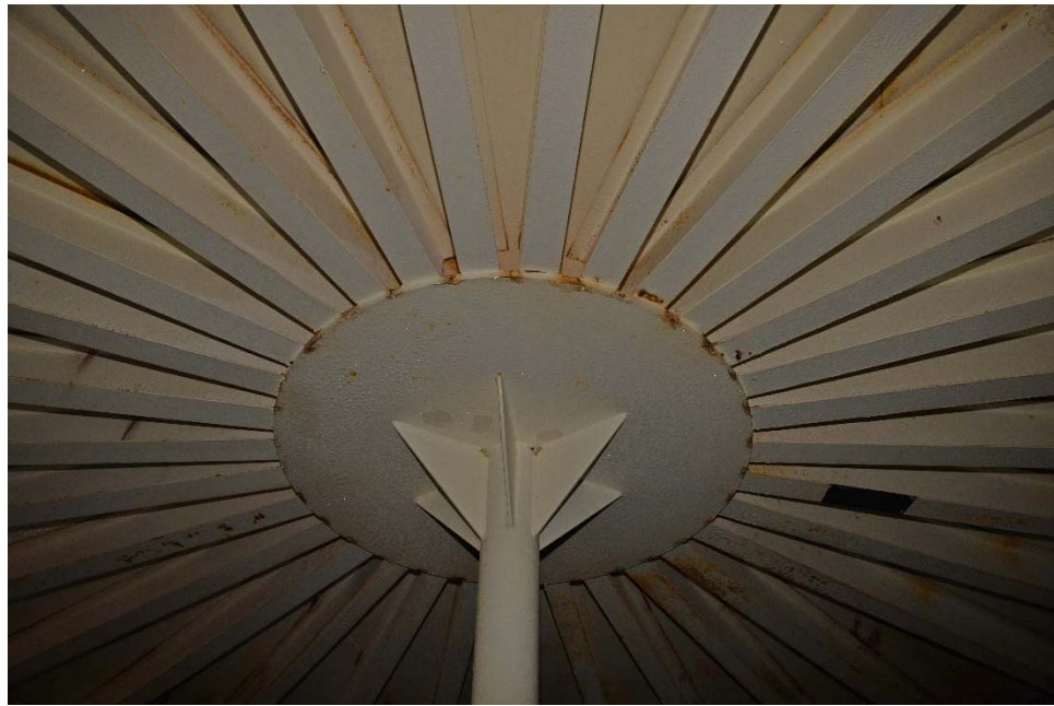
I-2 View of the center support structure, illustrating random minor corrosion on the lower rafter flanges and along the edge of the support plate.
