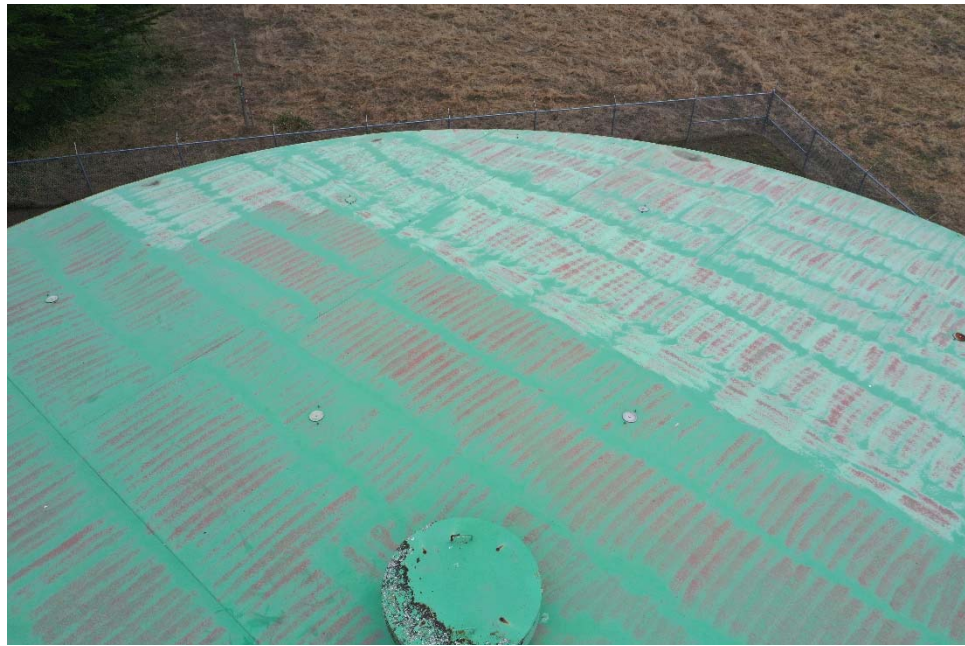
E-5 View of a portion of the roof, illustrating severe oxidation and fading of the paint system with exposed prime coat. Note pattern of exposed prime coat.
