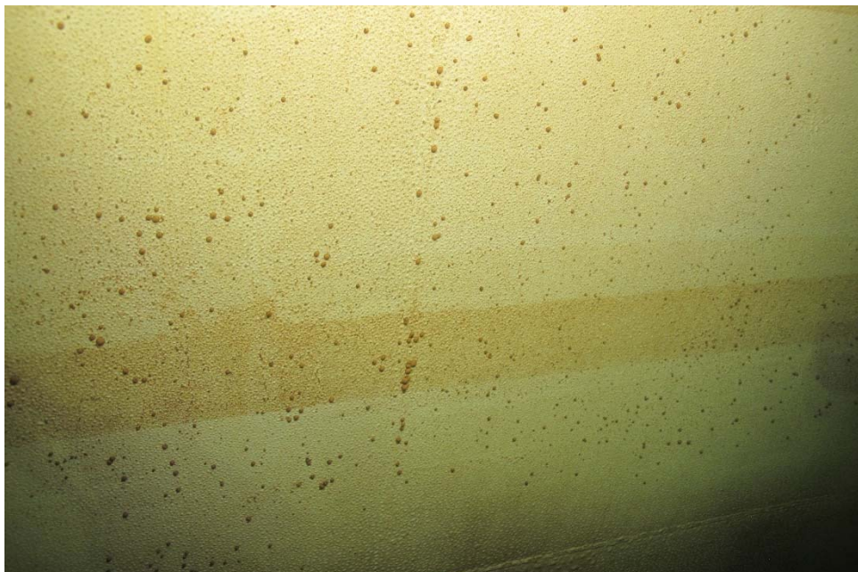
I-32 View of the shell, illustrating blistering of the coating system with numerous spots of corrosion.
