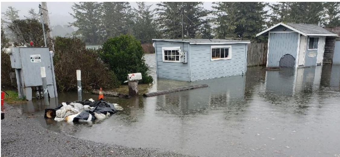
Figure 2: Flooding at the King Salmon Lift Station on January 3, 2022, as a result of King Tide coupled with storm surge.
