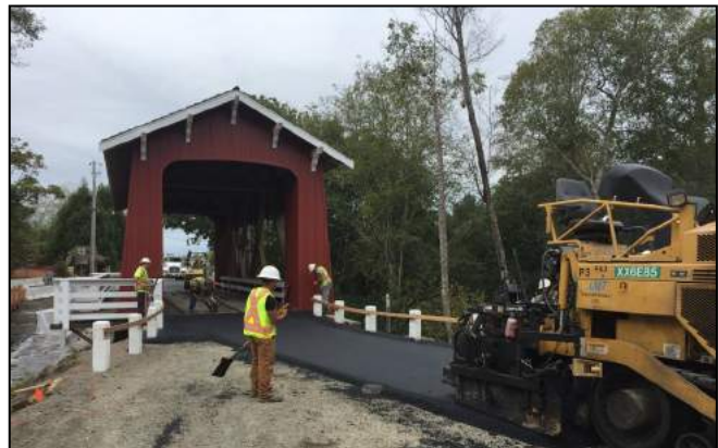
SHN provided construction management services for the County's Jacoby Creek Bridge rehabilitation.
