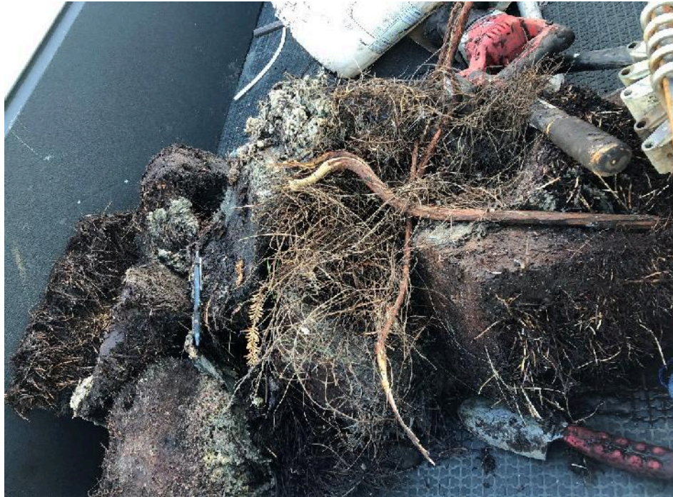
Figure 3: Root ball removed from sewer main near Sequoia discovered and removed on December 14, 2021.
