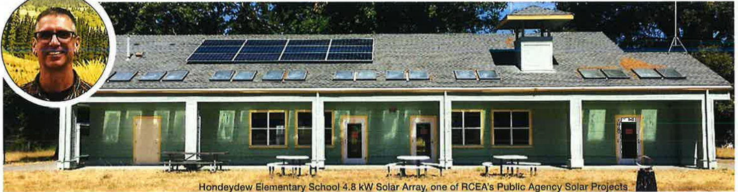
Hondeyde Elementary School 4.8 kW Solar Array, one of RCEA's Public Agency Solar Projects
