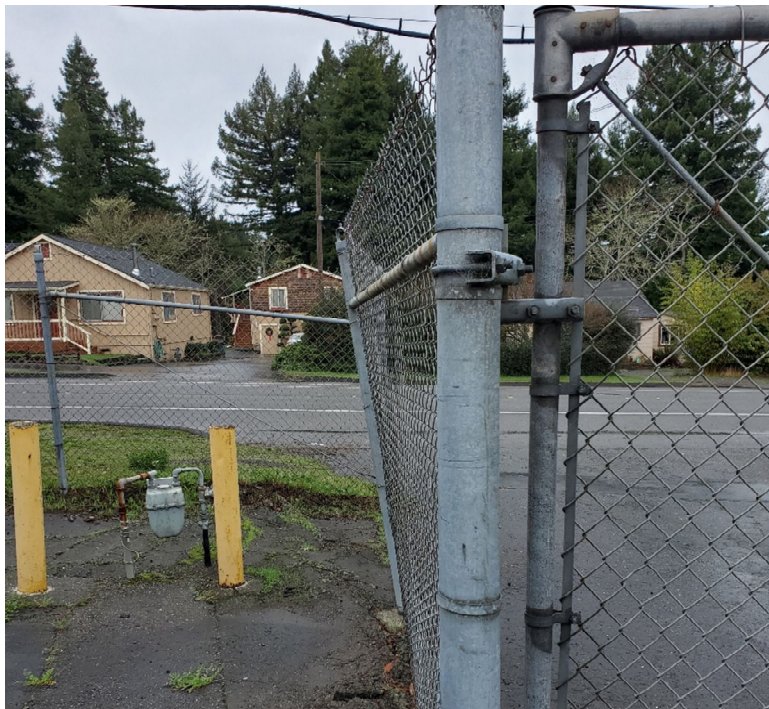
Figure 4: Looking west at south side of office building. Image shows damaged posts.
