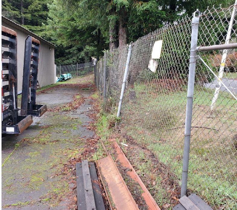
Figure 3: Looking south along the fence, south of the office building. Image shows damaged and leaning posts.
