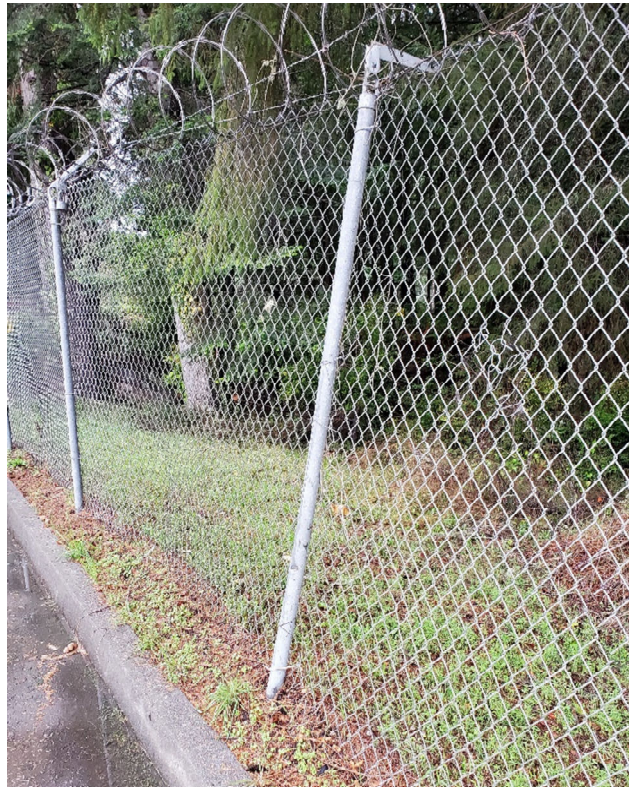
Figure 5: Northern portion of fence. Image shows damaged post as well as repaired damaged fabric resulting from a break-in.
